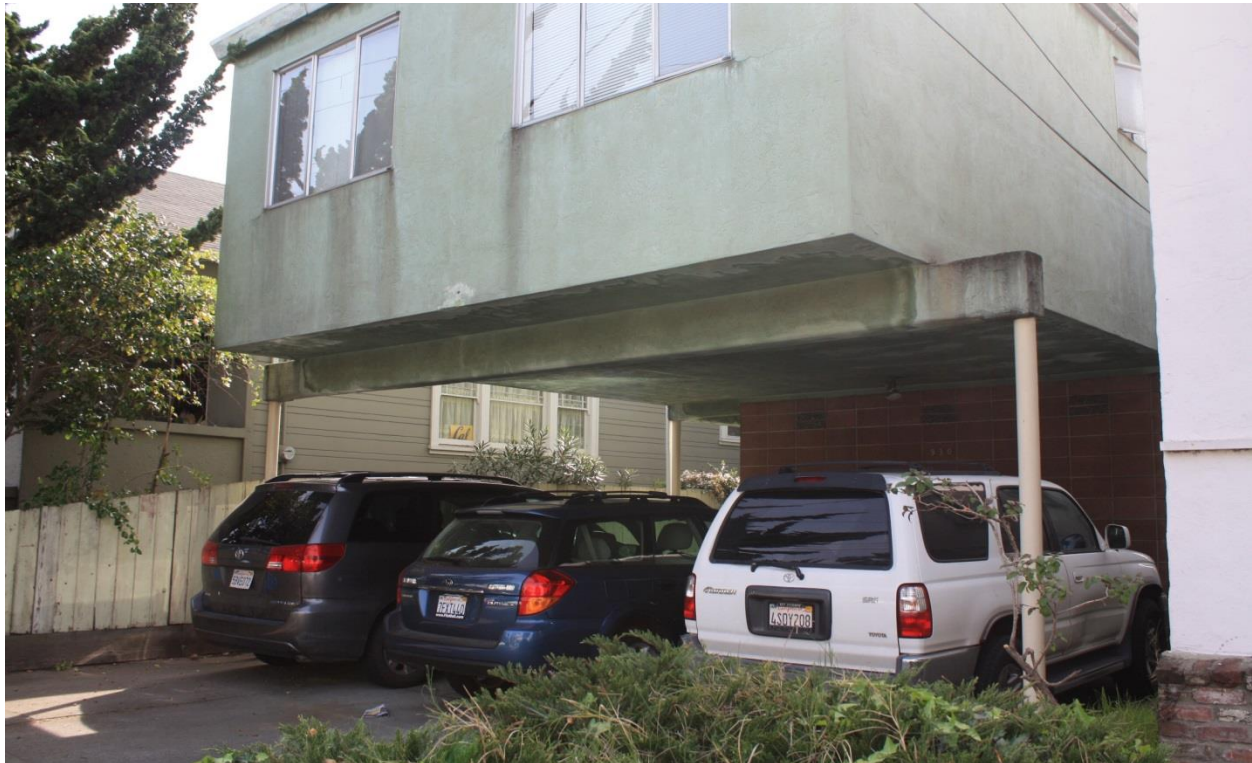
Soft-story buildings with “tuck under” parking are vulnerable in a major earthquake.
