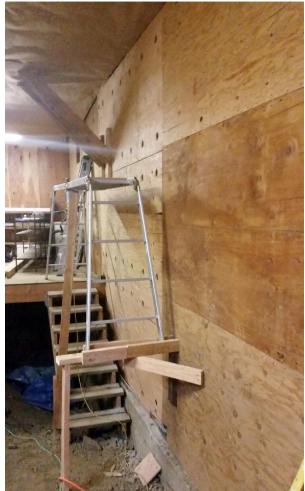
Installation of shear walls on a hillside home can help stabilize the structure during an earthquake.
