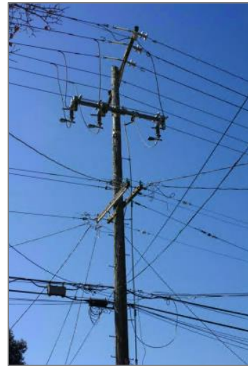
Overhead Utilities in Albany Photo courtesy of City of Albany General Plan
