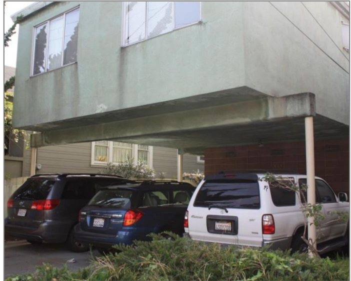
Soft Story Building in Albany Photo courtesy of City of Albany General Plan
