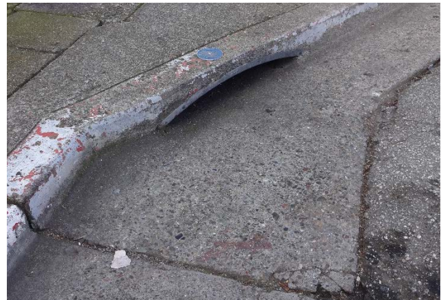
Figure B.19. Drainage infrastructure along Solano
