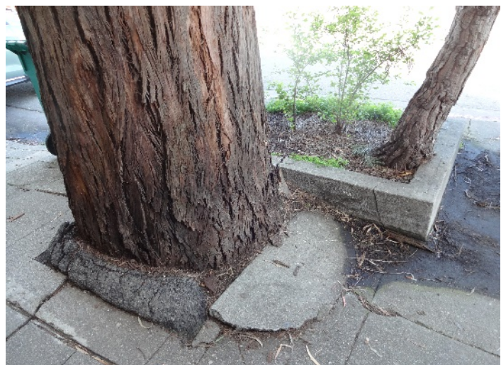
Figure B.6. Tree roots damaging the sidewalk.
