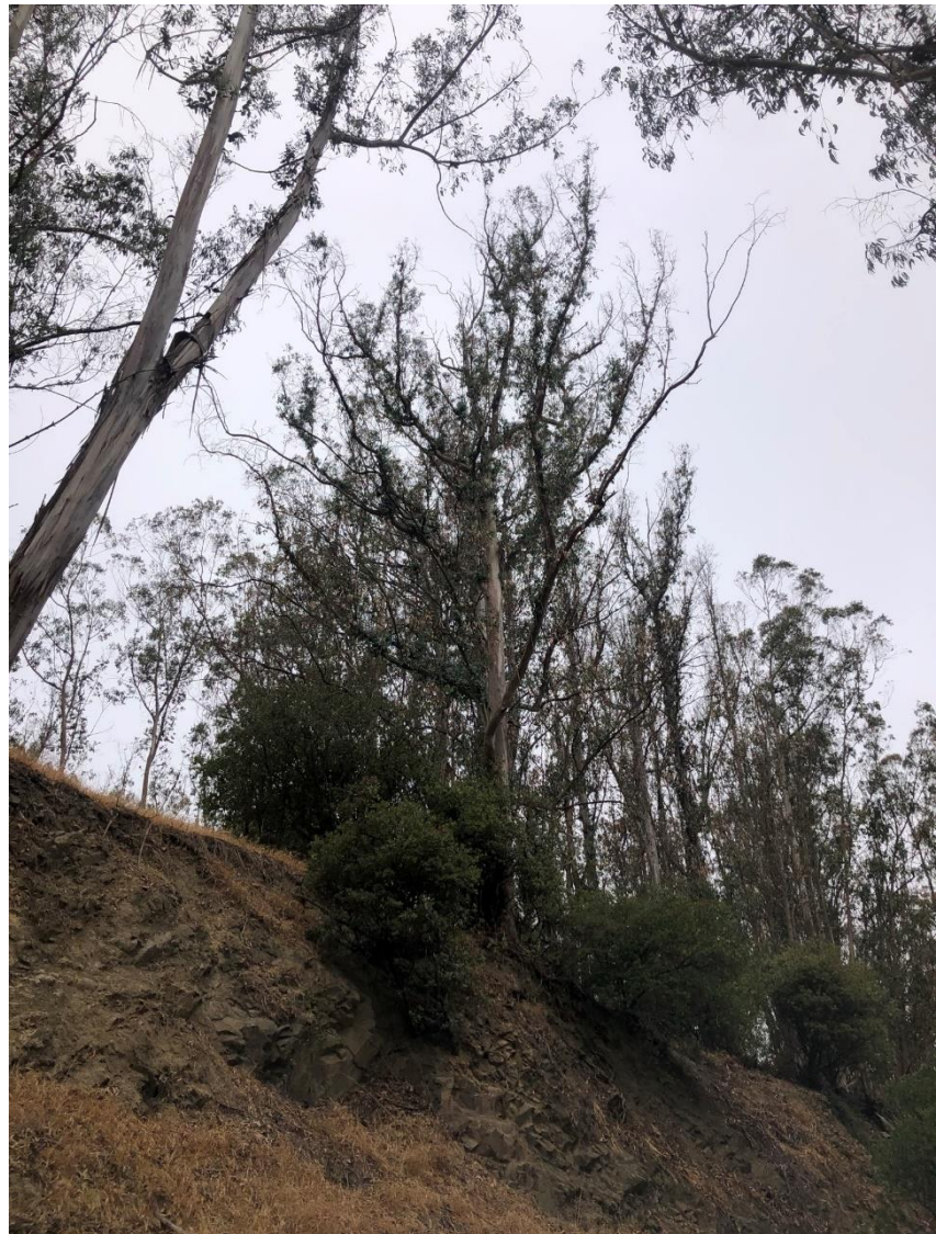
Photo 11. Photo right shows a tree in poor health condition at the edge of the slope. There is a higher risk associated with this tree due to the road and residences below.
