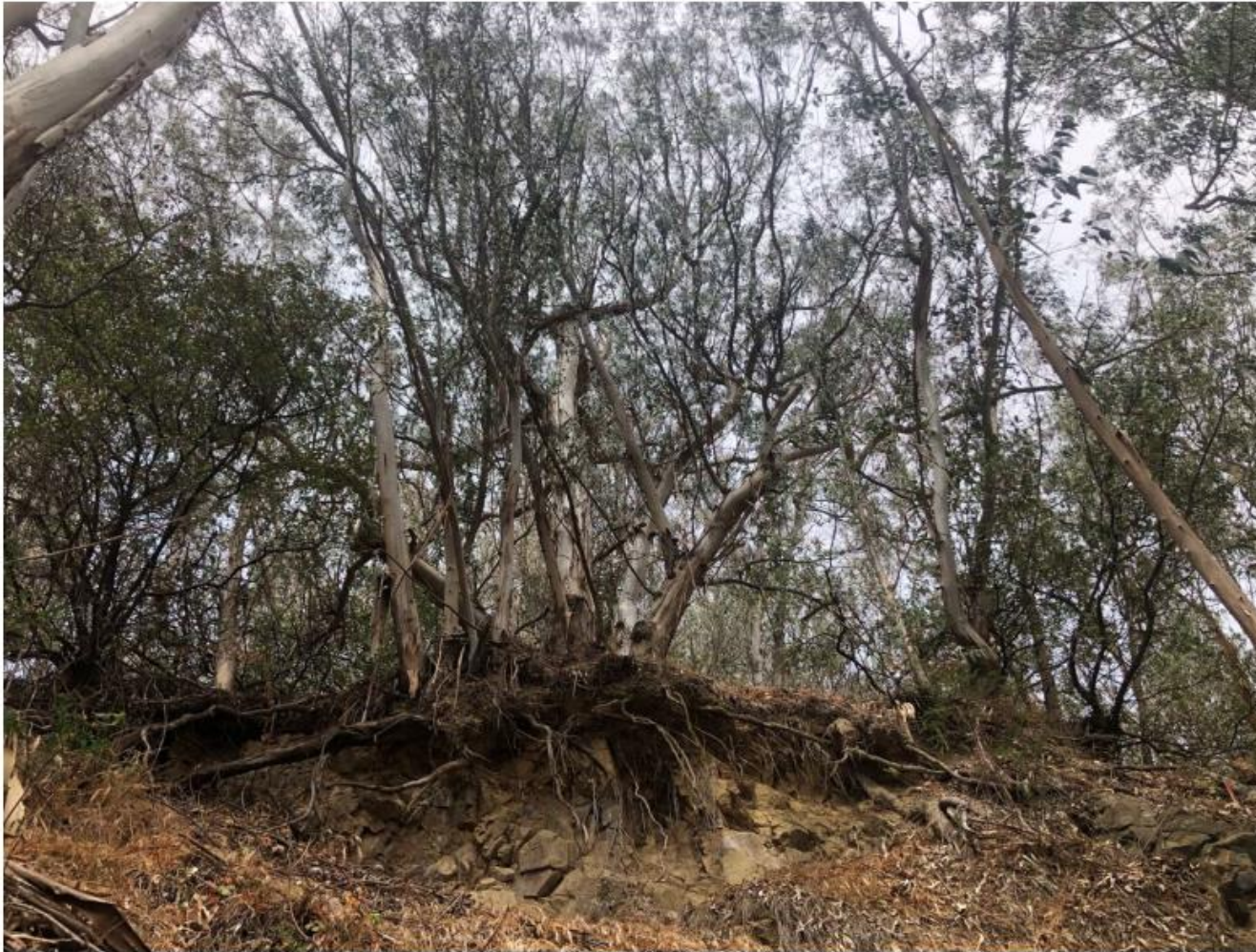
Photo 14. Photo above shows another example above of slope destabilization under trees.
